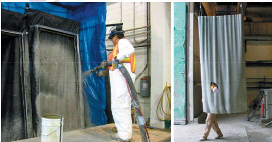
Fig. 14. Thin-shell precast wall panel created with sprayed concrete; photo: Mark West (C.A.S.T.) [49]
