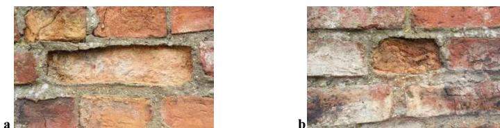
Fig. 1. (a) and (b) examples of frost damage.
