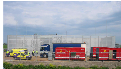
Figure 2a: Generator setup
