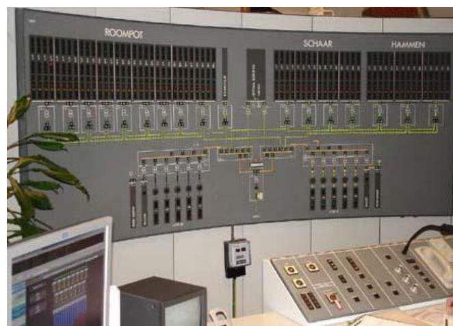
Figure 1.3: Picture of controlling panel sluices Eastern Scheldt
