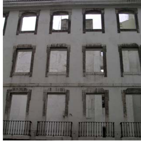
Fig. 5. Rehabilitation of a building Pombalino (XVIII century) in the city centre of Lisbon - Portugal, 2004
