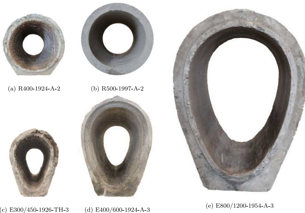
Fig. 1. A selection of unreinforced, used concrete sewer pipe specimens considered in the experimental program. Different surface conditions can be identified at the inner surface of the sewer pipes.
