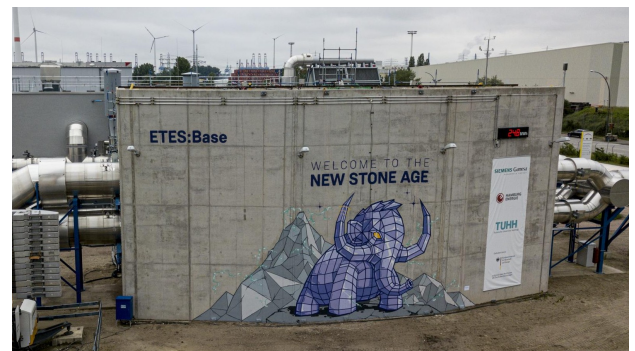
Figure 2: SIEMENS Gamesa's Carnot battery pilot plant located in Hamburg-Altenwerder (Gamesa, 2022)
