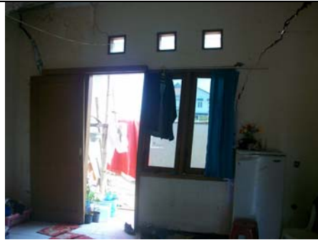
Door and window frame changes caused by the movements of land and building foundation.
