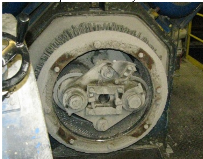
Figure 2: illustration of pelletizers installation with pellets coming out
