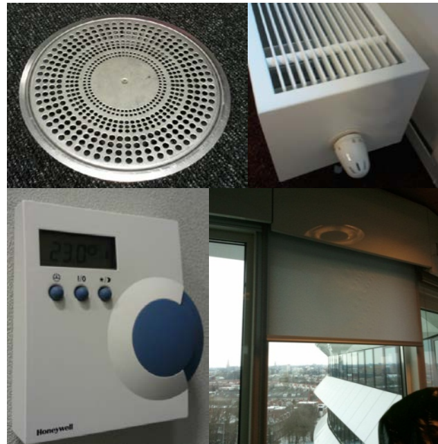
Figure 6. HVAC terminals and control systems in Building X
