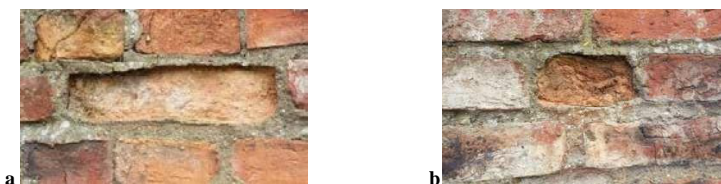
Fig. 1. (a) and (b) examples of frost damage.
